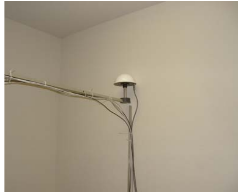
Figure 5. Position of H-field antenna for indoor tests in Cedar Park, Texas. The antenna was situated next to a wall and away from windows.
