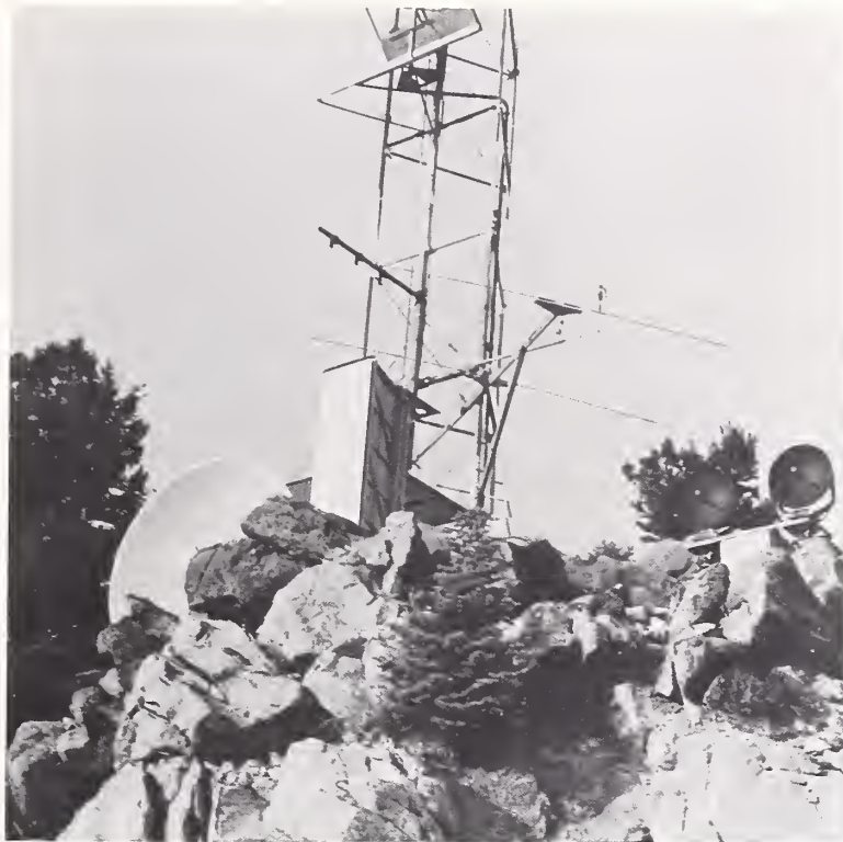
Lower section of antenna tower at "summit site," Cheyenne Mountain. Also, visible are antennas installed later for additional research projects.
