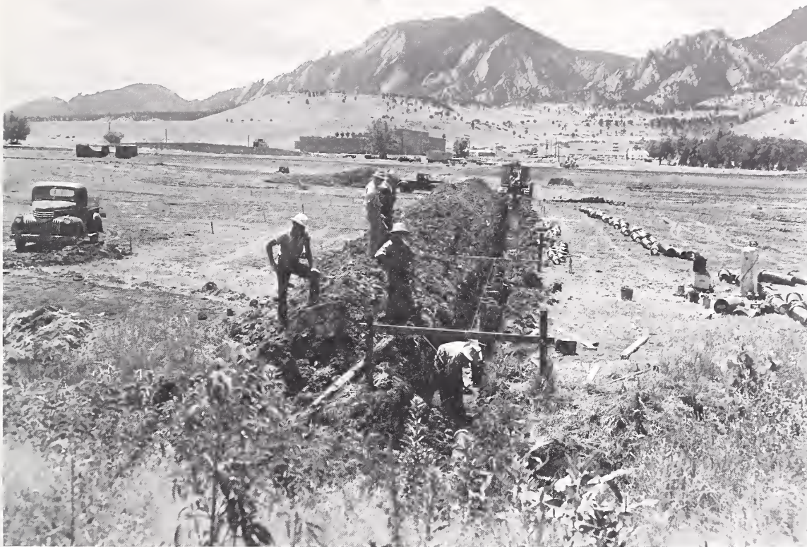
The site of Boulder Laboratories as it appeared on July 15, 1952, a few weeks after ground was broken for construction of the Radio Building. The tiled drain in foreground is located just to the north of the auditorium section of the Radio Building that was completed in the spring of 1954. In mid distance can be seen the Liquefier Building and the Camco Building, both constructed during 1951. Occupying the horizon at center is Bear Mountain, that provides a spectacular backdrop for the Boulder Laboratories in a southwesterly direction. Buildings of the National Center for Atmospheric Research now occupy the hilltop (known as Table Mesa) to the left and front of Bear Mountain.
