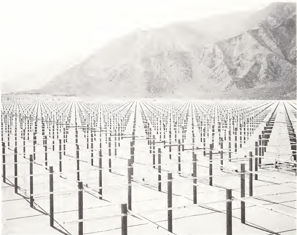
Dipoles by the thousands (9216 crossed pairs of half-wave dipoles)—covering an area of 21 acres—that serve as a huge antenna for a scatter radar installation. Construction of the facility, known as the Jicamarca Radar Observatory, began in January 1961 at Jicamarca, a site east of Lima, Peru, located near the geomagnetic equator. This venture into new realms of radio research of the ionosphere was a cooperative project of the Central Radio Propagation Laboratory and the Instituto Geofísico de Perú.
