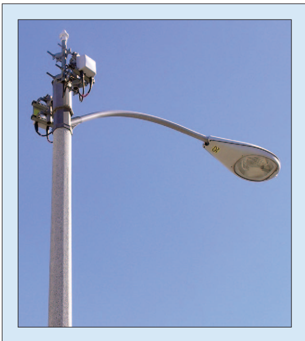
Fig. 3. GPS antenna (top of pole) deployed for mobile phone network.
